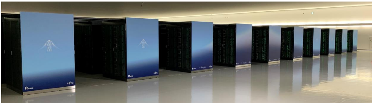
Figure 2 : The Fugaku system at RIKEN (Japan)
