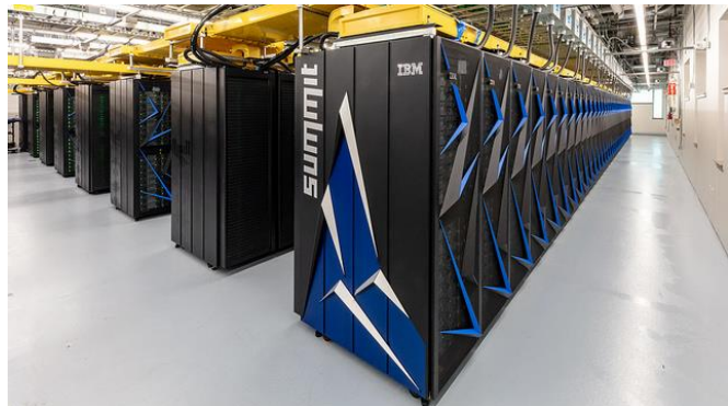
Figure 3 : The Summit supercomputer installed at Oak Ridge
